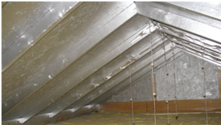
Figure 5 Test attic with liquid applied low-e coating on roof deck and rafters.
