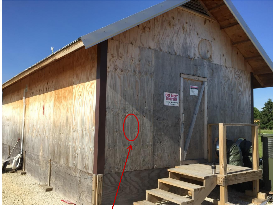
Temperature sensor and HFT location
