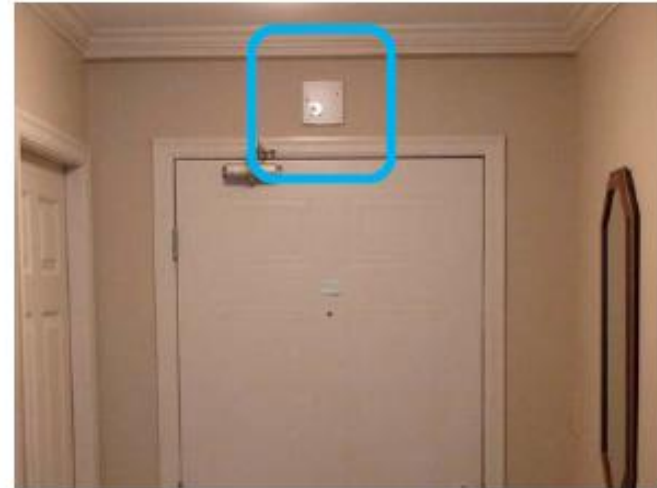
Figure 7-24: Typical data acquisition unit installed above a suite entrance door
