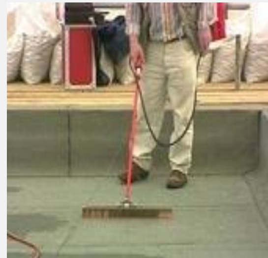
High Voltage Dry Scan
