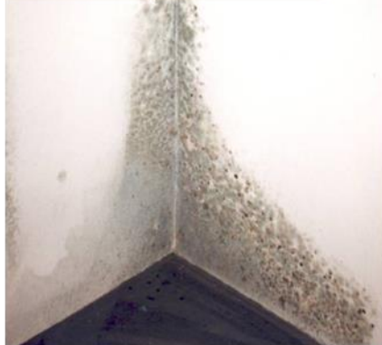
Cold surface behind cupboard ( Germany )
