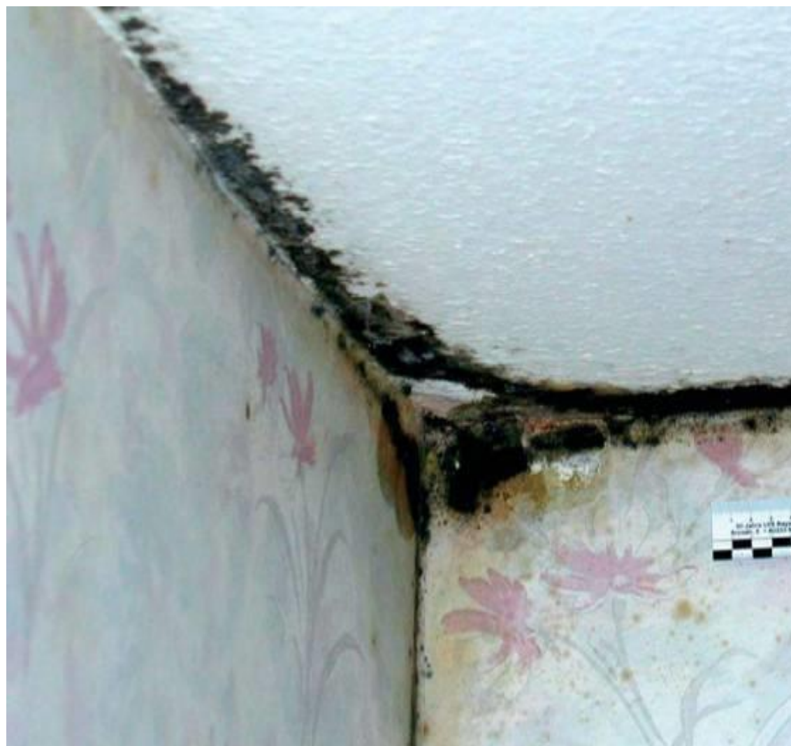
Mould at corners and edges
