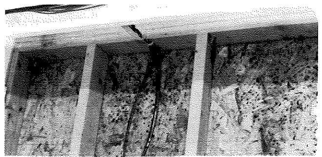
Figure 12 Fungal growth at top of cavity with faced insulation.
