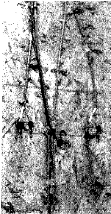
Figure 11 Rust on metal fasteners in cellulose cavity without vapor diffusion protection.
