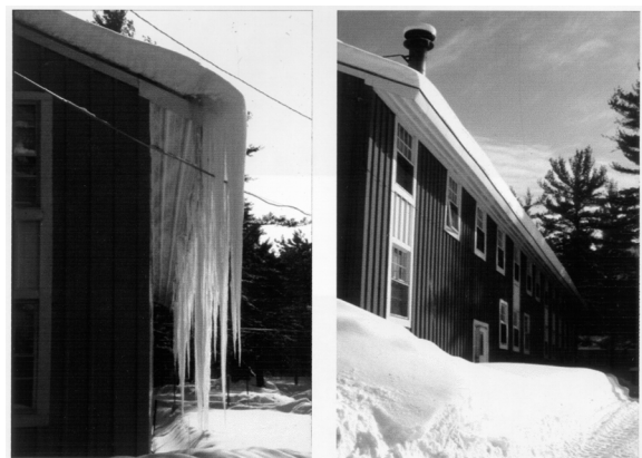
Figure 1 Two identically constructed roofs photographed at the same time. The one on the right, with no icings, was unheated.
