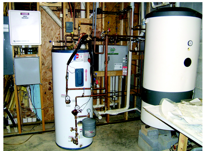
Figure 9 Prototype DHW Heat Pump System
