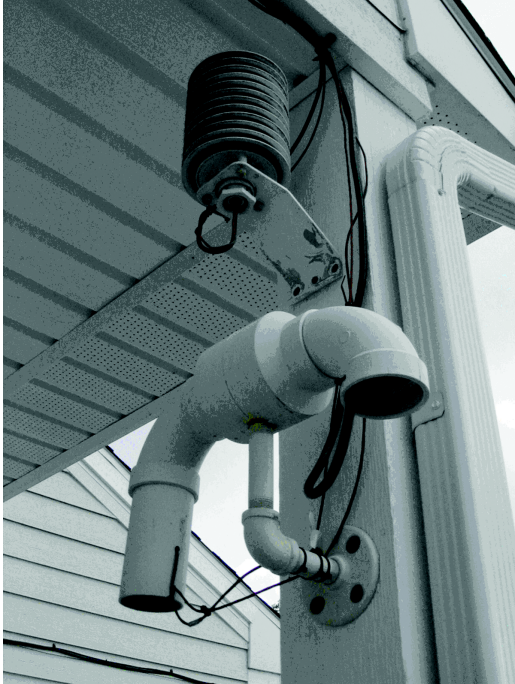
Figure 4 Outdoor temperature and humidity sensors.
