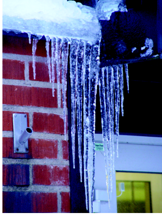
Figure 8 Icicles at roof eaves.
