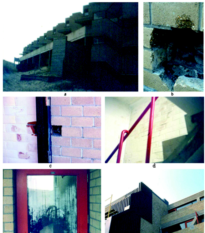
Figure 6 Hotel at the Belgian coast: (a) the building, (b) tray short-circuited by mortar debris, (c) lack of a watertight layer where the veneer touches the inside walls, (d) wet inside leaf, (e) surface condensation on double glazing, (f) final retrofit
