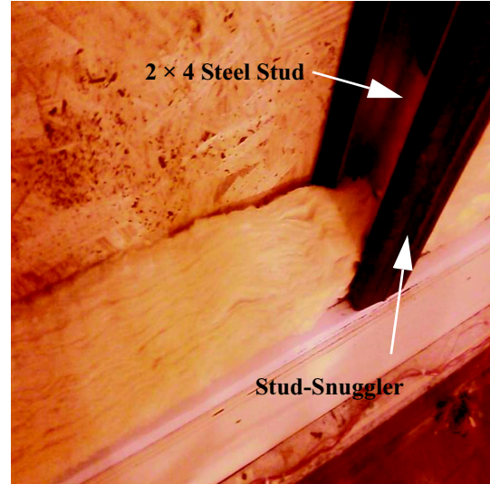
Figure 2 Application of the stud-snuggler foam profile over steel stud and installation of R-19 fiberglass insulation.
