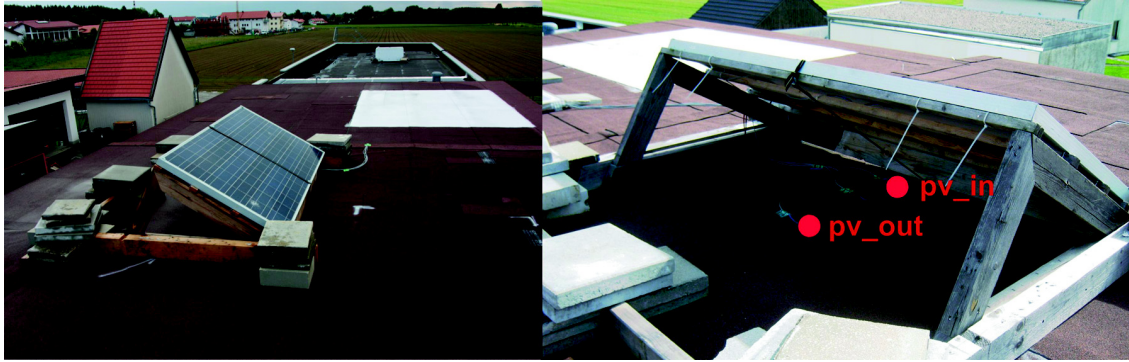
Figure 2 The solar panel and the sensor positions.
