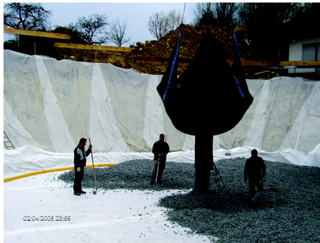
Figure 8 Placement of cellular glass aggregate with the help of a crane and a sheet with a plug valve onto which the cellular glass is unloaded from the truck. (Reproduced by permission of Misapor AG.)
