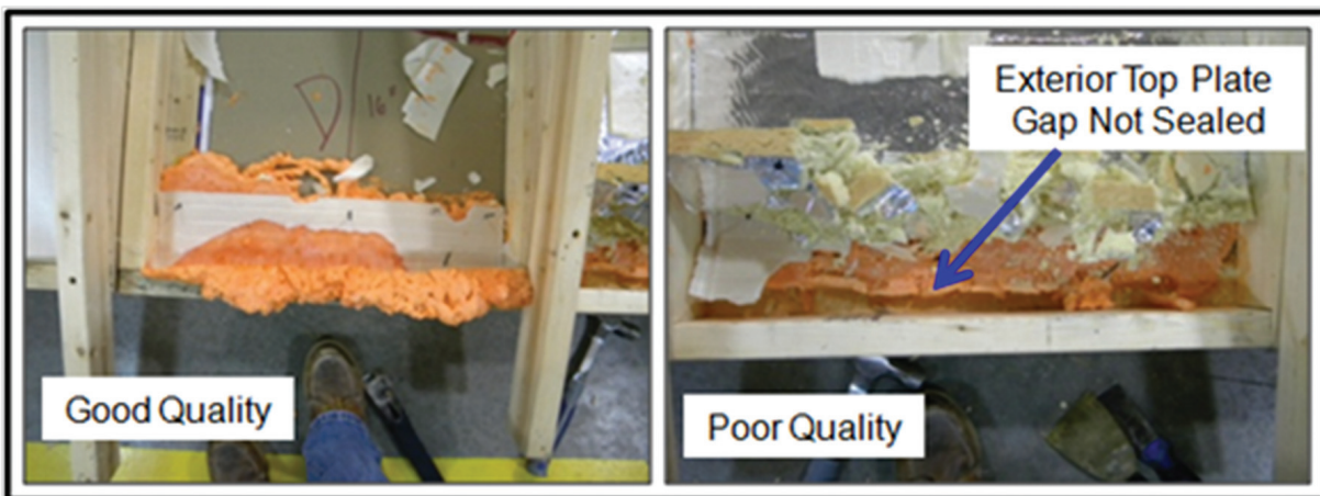
Figure 11 Examples of good- and poor-quality foam sealant installations using techniques 2a and 2b, respectively.
