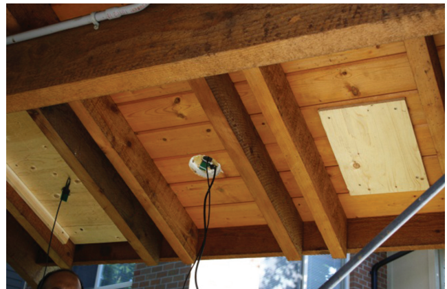
Figure 7 Control assembly sensors.
