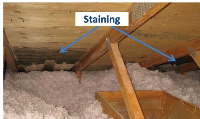
Figure 1 Staining (mold) at soffit vents in a recently constructed wood-frame project.
